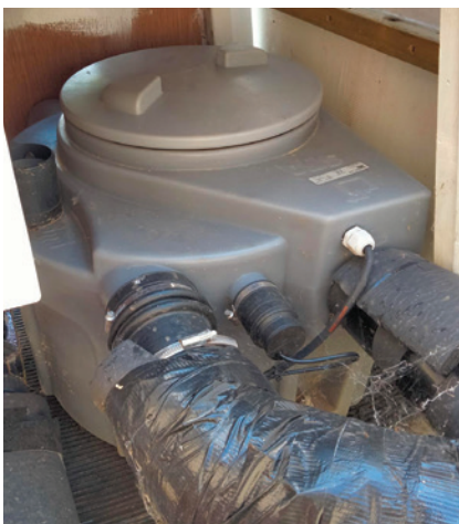
The Saniflos 110 takes the waste from the internal pumps and discharges it through small bore pipework up the hill to the mains drains
