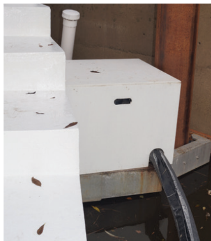
The Saniflos 110 is installed in a box adjacent to the house and floats up and down with the house as the tide moves
